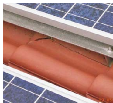
Abb. 5: Ziegelbruch Figure 5: Broken tiles
